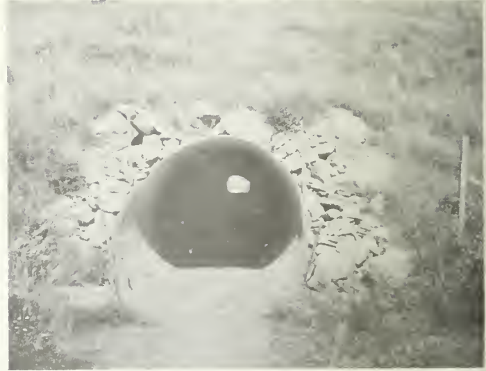
SOUTH ENTRANCE; Notice bulge
